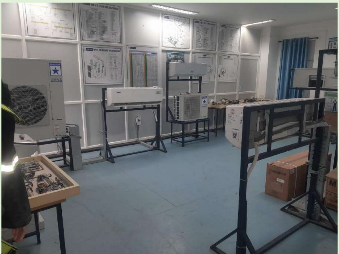
Equipment's in HVAC-Hands on Training Centre procured through Industrial Collaboration [Blue Star Ltd]
