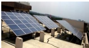
25 kWp PV Plant installed by Alumni
