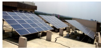
25 kWp PV Plant installed by Alumni
