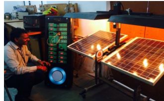
PV Training and research Experimentation facility
