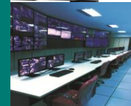
Centralized Network Control Room
