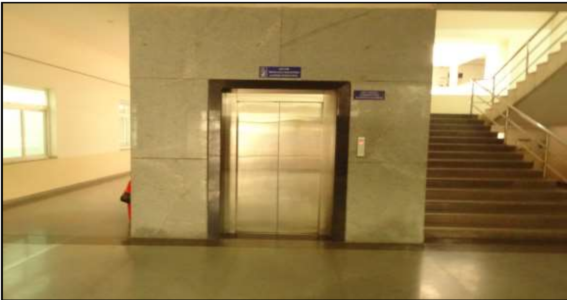
Lift 6 in Yogiah Naidu Bhavan of 12 Persons capacity
