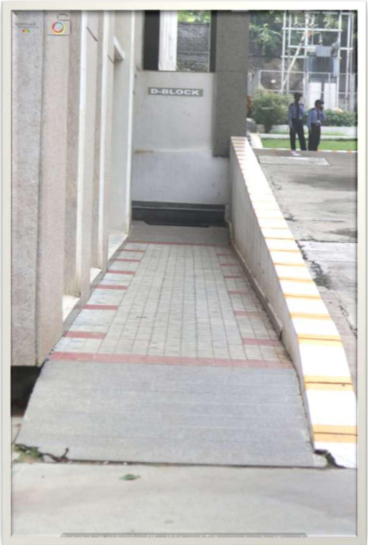
Ramp & Rail in Yogaiah Naidu Bhavan (CE, ME and AE) – D Block
